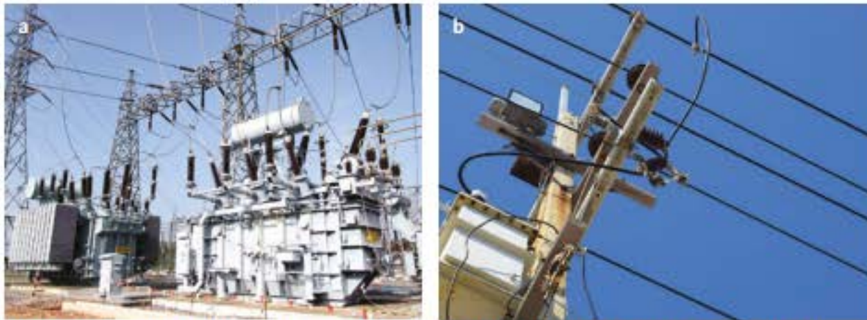
FIGURE 6.4.1 (a) Transformers at an electrical substation. The substation takes electricity from the distribution grid and converts it to lower voltages used by industrial or residential equipment. (b) More common are the smaller distribution transformers found on every suburban street. See if you can locate at least one on your street.
